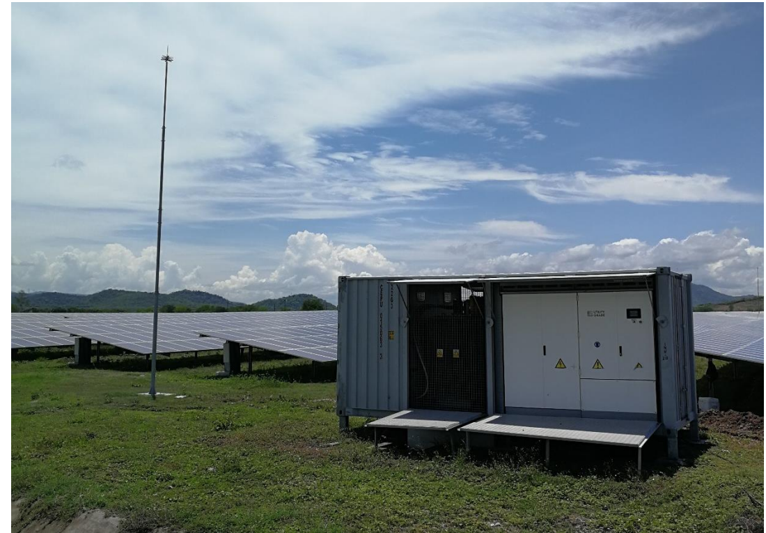
ESE lightning rod in a free-standing pole
