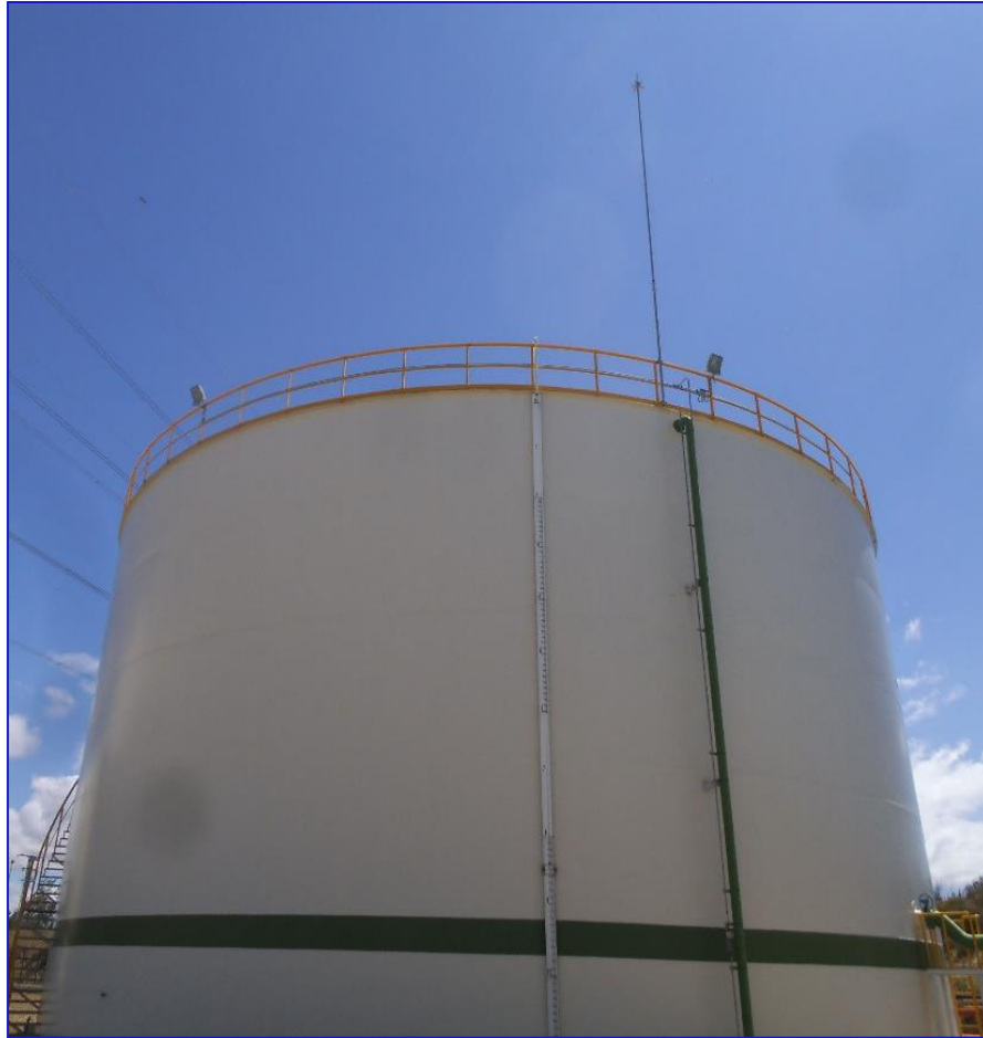
Lightning rod in a tank
