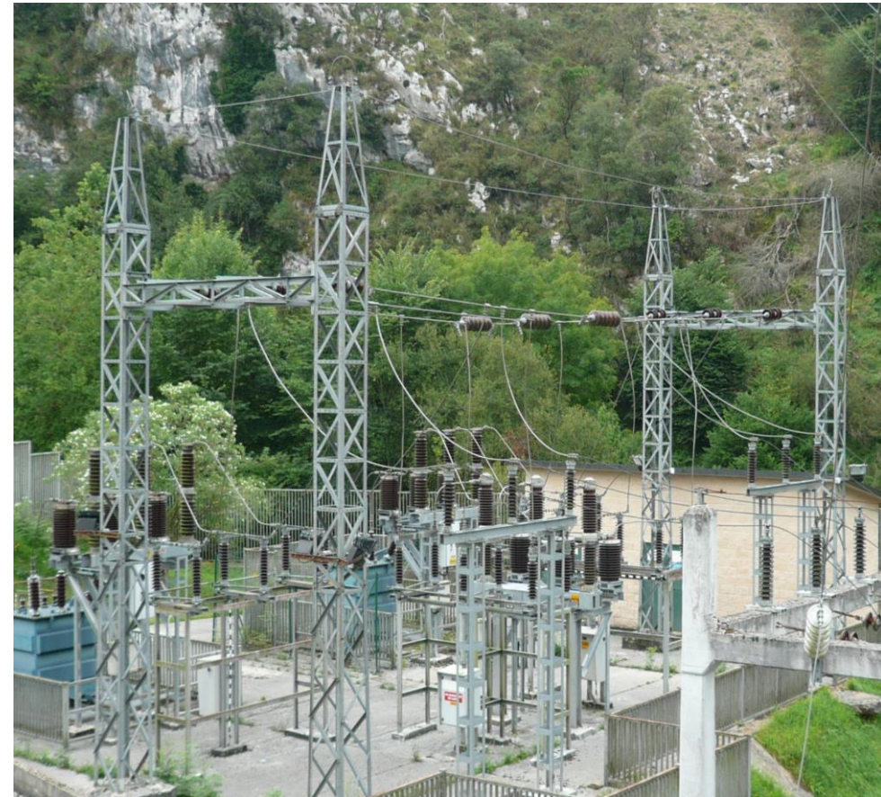
Catenary or overhead cable
