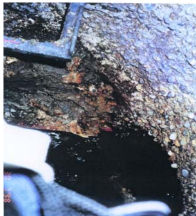
Fig. 5: Biogenic sulphuric acid corrosion in a manhole
